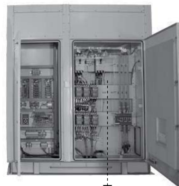
Electrical and control panel
